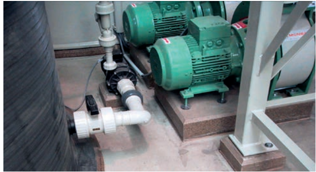
Polly-concrete bricks as pumping equipment foundation
