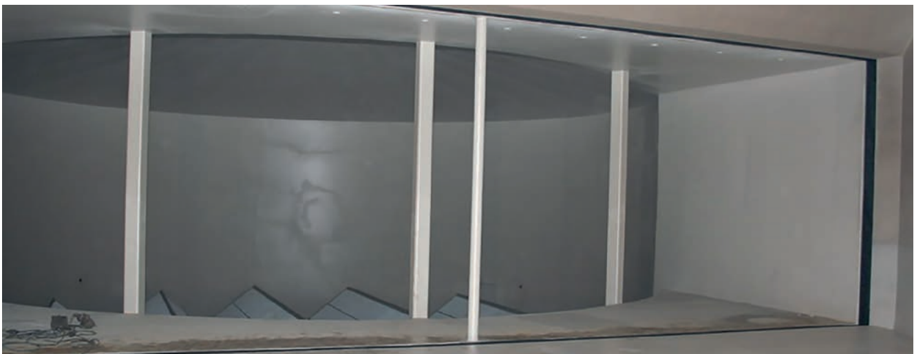
Coated clean gas duct
