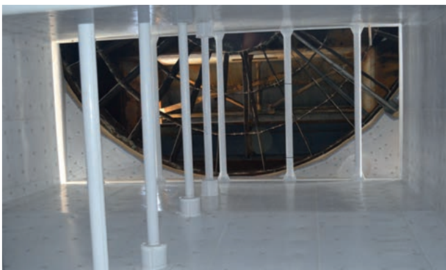
PFA lining in a raw gas duct
