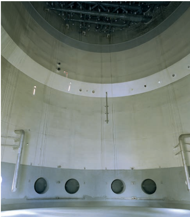
Lined flue gas scrubber
