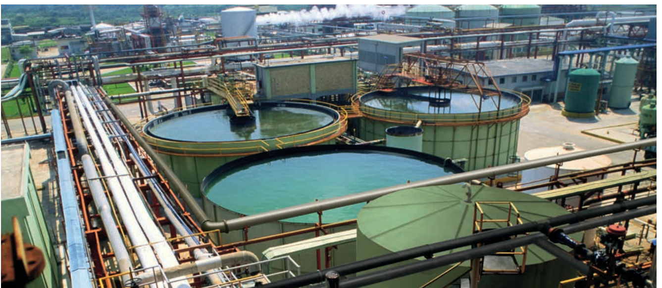
Rubber-lined sedimentation tank
