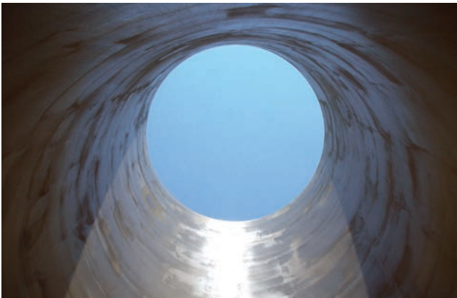
With COROFLAKE 23 coated chimney
