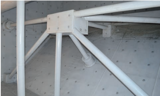
PFA lining in a raw gas duct
